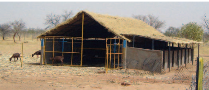
This goat shelter was built with local materials and a metal frame. 8 birthing stalls are on its west side.
